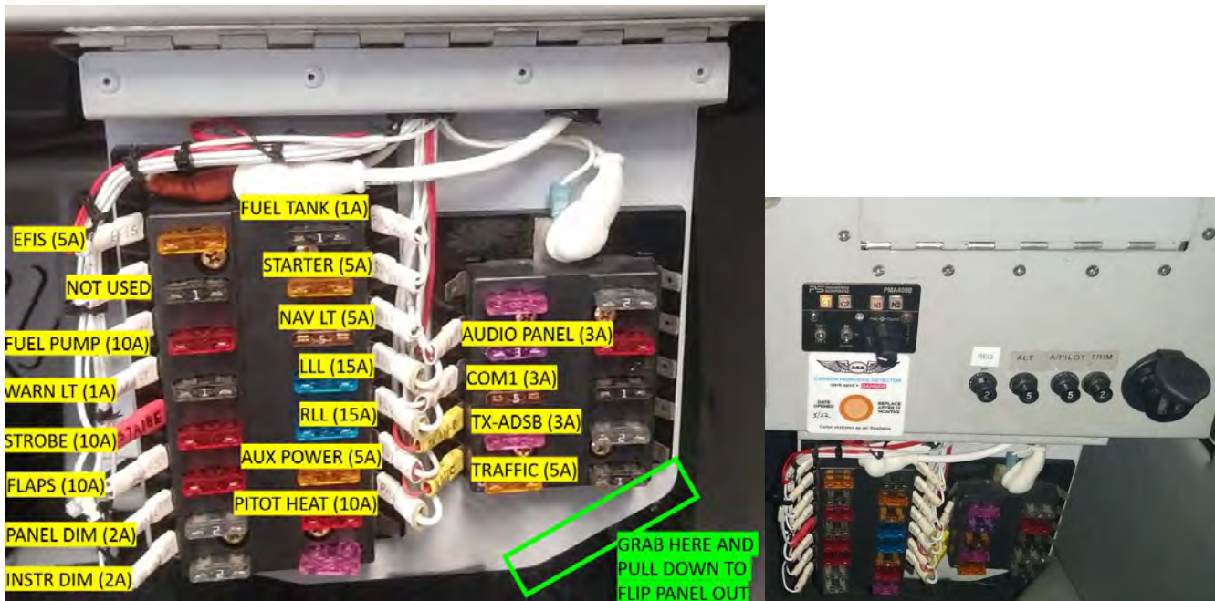
Figure 15 – LEFT: The fuse panel (flips out on passenger side from under dash).
